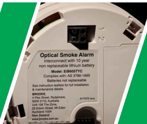
10-year lithium battery alarm
